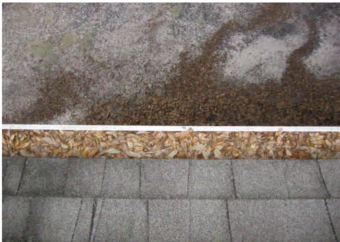
Figure Set 4 - The gutters on the composition shingle roof should be cleaned and serviced to drain properly
